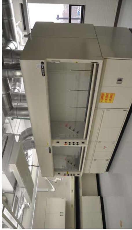
Phase Two - Carbon Materials and Solar Array Laboratory
