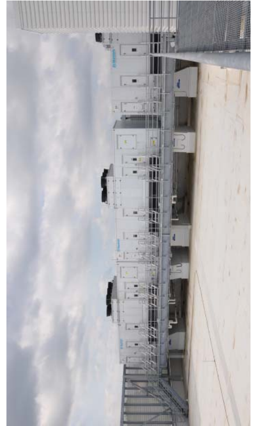
Indirect Evaporative Cooling Units support the whitespace
