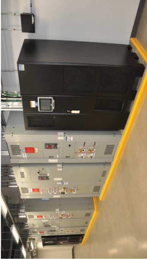
Uninterruptable Power Supply provides additional 400KW
