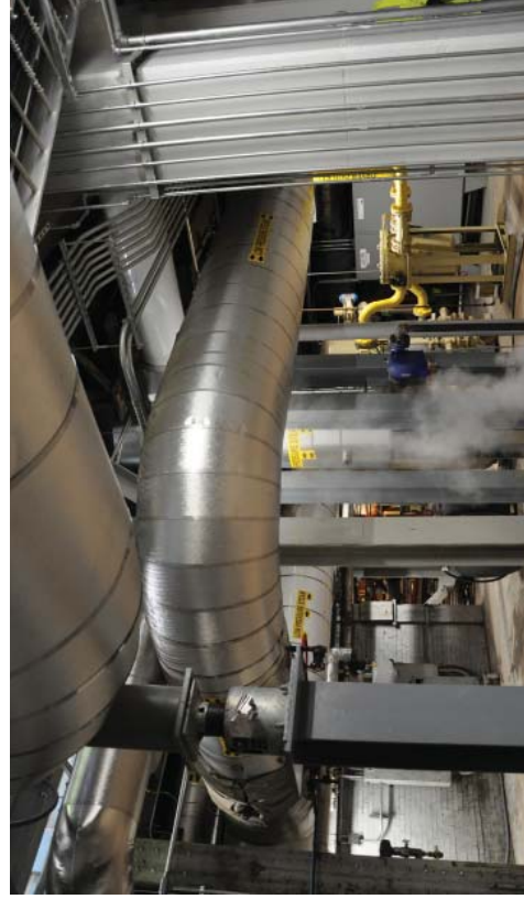
High/Low Pressure steam lines below the new turbines
