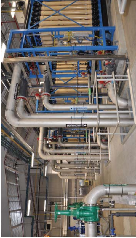
Microfiltration area treats bacterial/protozoan contaminants
